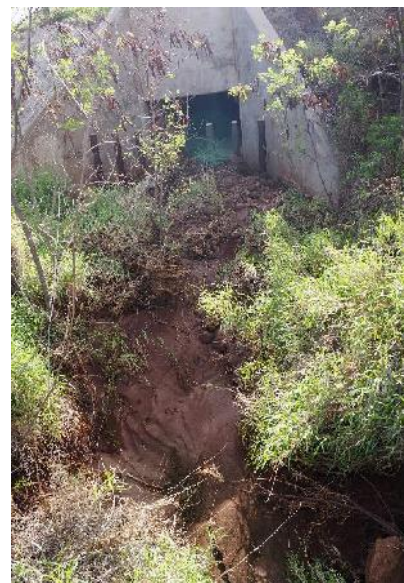
Evidence of sediment laden stormwater
