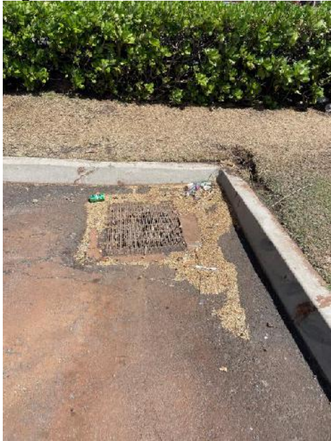
Figure 17. Storm Drain BMPs
