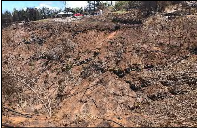
Picture 10. Slope instability observed in the Kula Fire (USDA FS)
