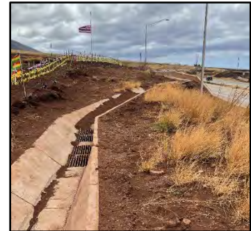
Picture 18. Windblown ash and sediment in a drainage ditch on the Lahaina Fire (USDA FS)
