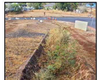
Picture 19. Drainage ditch below the Lahaina Fire that needs cleaning (USDA FS)
