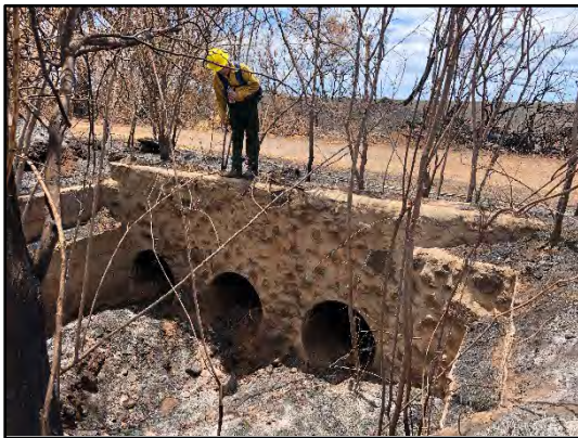
Picture 9. BAER team member assessing culvert condition in the Lahaina Fire (USDA FS)
